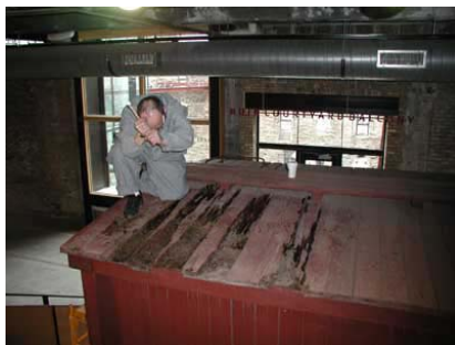
Figure 10: Detail of roof board stabilization in progress. The darker areas show where the liquid epoxy was used.
