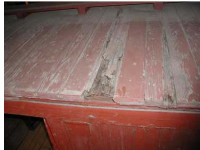
Figure 9: View of deteriorated roof boards before treatment.
